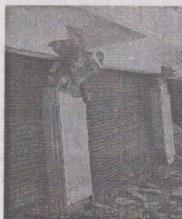
Fig.2 Column failure (2001 Bhuj earthquake)
